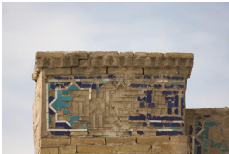
Figure 2: Damaged tiles on the top of a column of the mosque Khoja Zainuddin in Bukhara, Uzbekistan, Badr et al. (2010).
