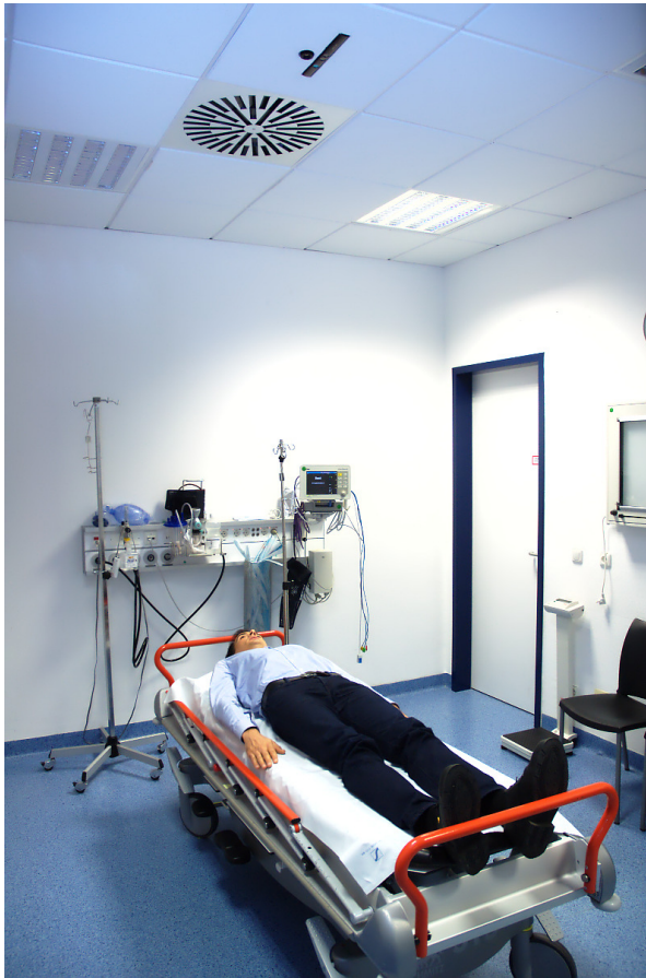
(a) Trauma room with sensors integrated into the ceiling
