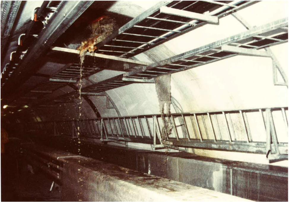
Fig. 4.11. Failure of tunnel concrete lining in 1990.
