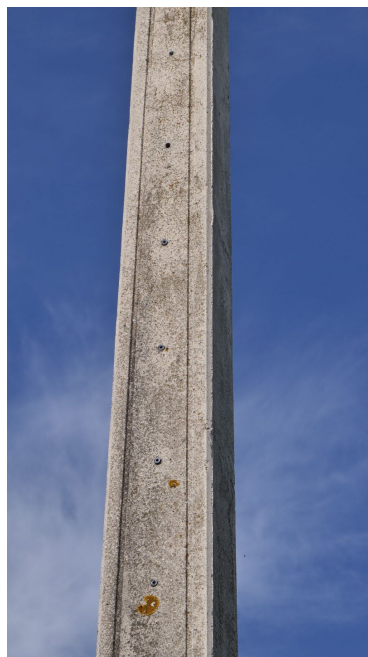
Figure S4: Power pole with closed entrances probably due to maintenance work of the electricity company. The bees cannot enter the hollow pole anymore to build a nest inside the cavity.
