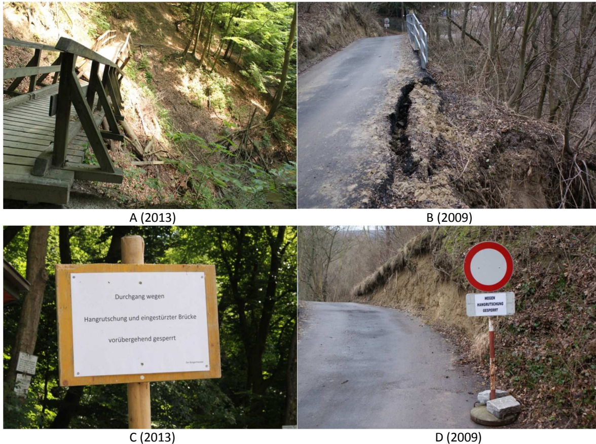
Figure 1-1. Damage caused by mass movements in the Northern Vienna Forest: (A) destroyed bridge in the Hagenbach Valley, (B) damaged road in the study area, (C) announcement “No trespassing because of a destroyed bridge”, (D) No vehicles: “road closed because of landslide”. Photos: (A, C) B. Neuhäuser, (B, D) Department of Torrent and Avalanche Control.
