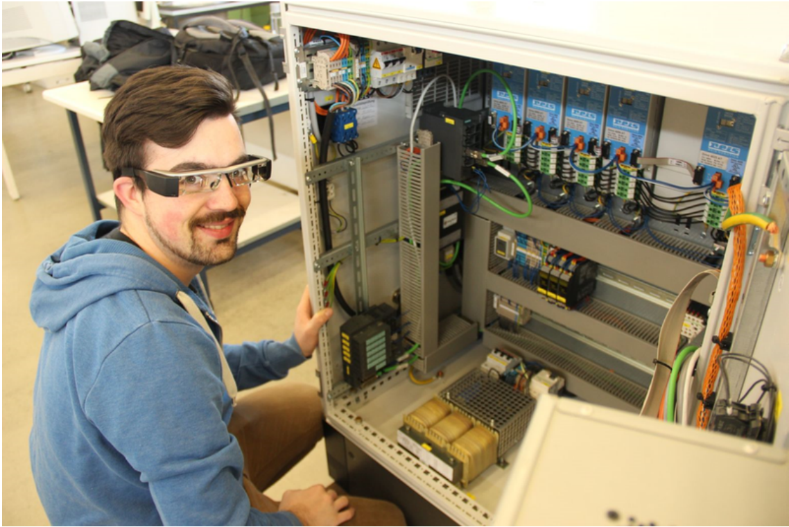
Figure 4.22: The switch cabinet with integrated servo amplifiers (blue)
