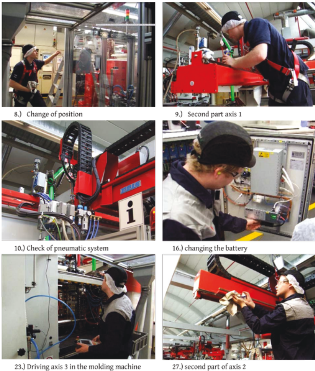
Figure 4.5: Maintenance of industrial robot (visualization part 2)
