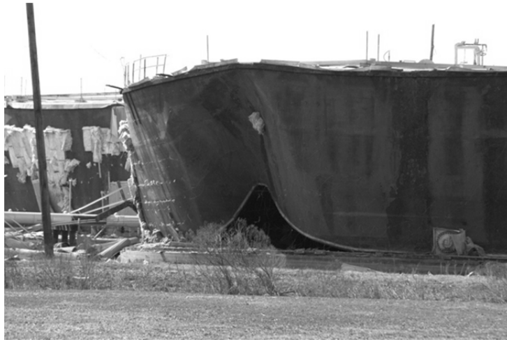
Figure 6: Tank damages after Hurricane Katrina in Louisiana 2005 (M. NAUMAN, FEMA photo library ID No. 20548)
