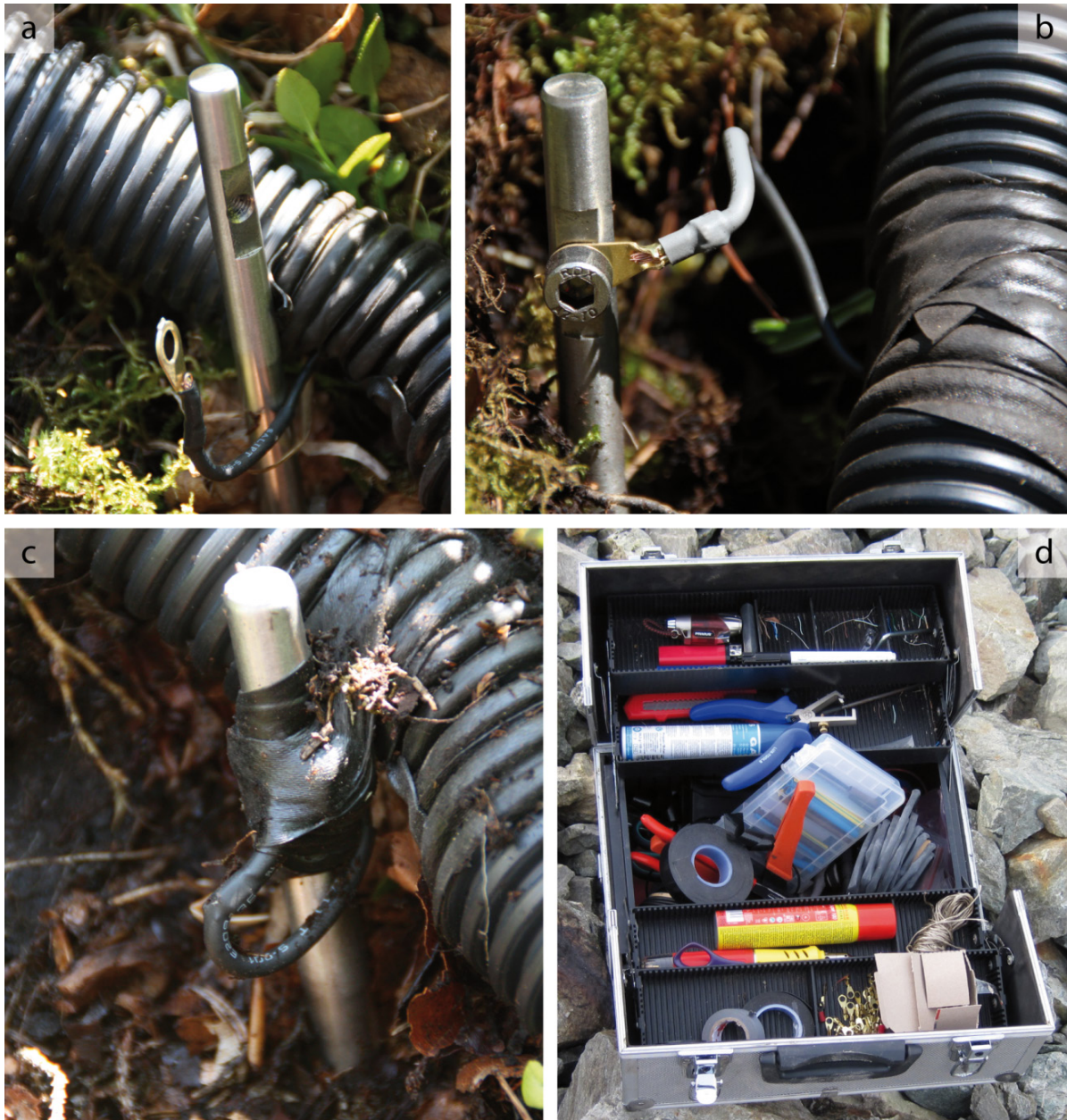
Figure 7.2: Installation of the fixed ERTM array, with connection and isolation of transitions between cable and electrode (a-c) and basic tools for the installation (d).
